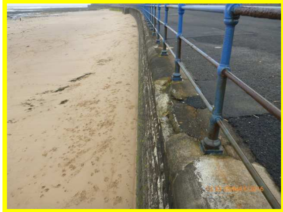
Local damage to wall crest (/C0303C01)
