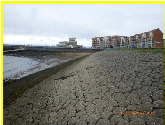
Local settlement of concrete blocks (/C0401C26)
