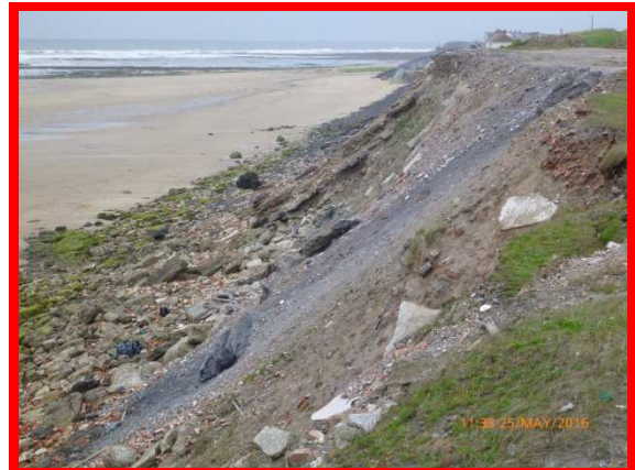
Erosion of made ground slope to south of former gabion structure (/C0302C02)
