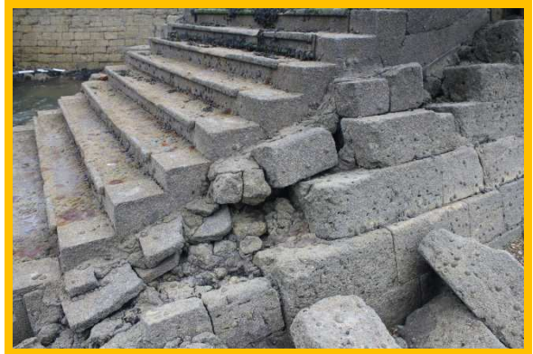
Damage to steps at former passenger ferry landing (/C0401C35)
