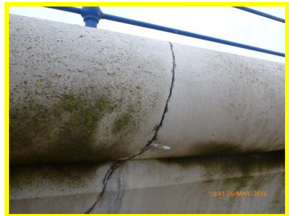
Crack in concrete cope. Note previous repair/fill now failing (/C0501C05)
