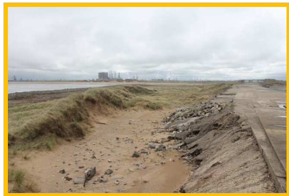
South face of North Gare Breakwater. Dune field in lee of structure (/C0503C01)
