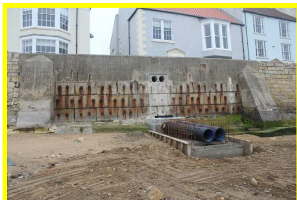
Concrete section of wall, ongoing construction of outfall. Significant corrosion/rust staining previously observed (C0401C35)
