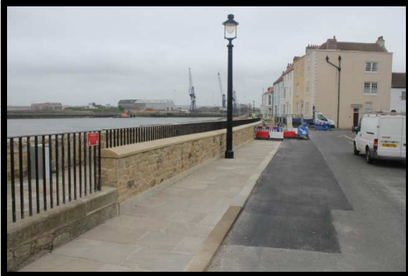
Recently completed masonry wall and walkway to rear of seawall along Northgate. Works continue in background. (/C0401C35)
