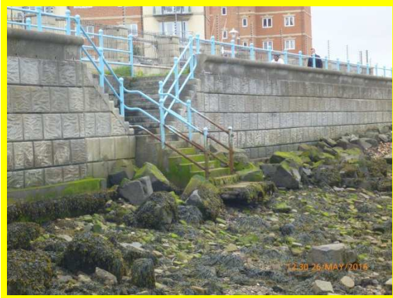
Undercutting of access steps (/C0401C27)
