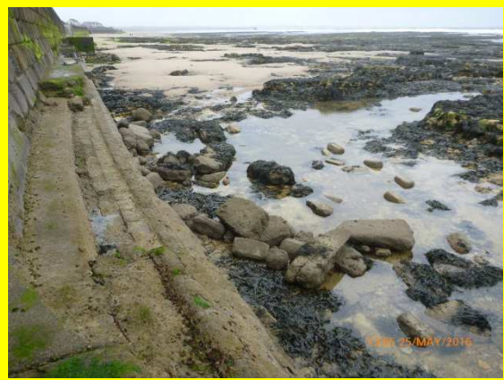
Abrasion of concrete toe protection. Displaced concrete on foreshore (/C0303C02)
