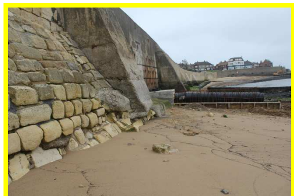
Open jointing in lower masonry courses. Local undermining of concrete buttress (C0401C35)
