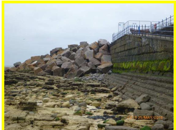
Rock armour forming temporary construction access south of Broad Field Road access ramp (/C0303C02)
