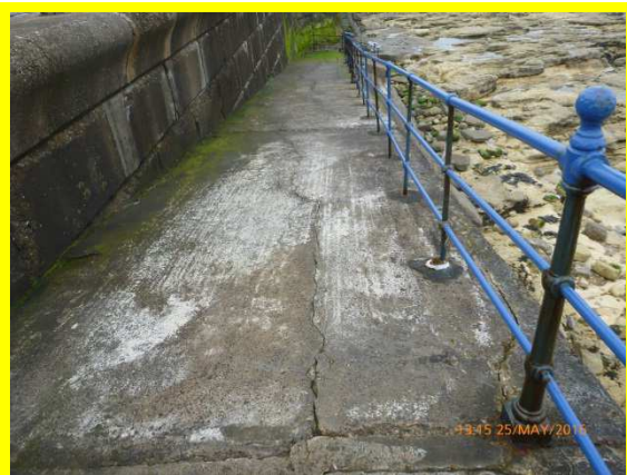
Longitudinal crack in Broad Field Road access ramp (/C0303C02)
