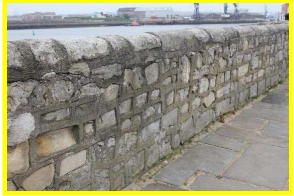
Previous repairs. Mortar used in repointing appears to be stronger than masonry and now stands proud of the stone (/C0401C35)
