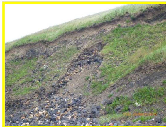
Local slope failure (/C0302C03)
