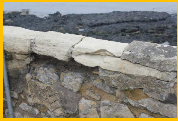
Missing masonry at crest (/C0401C35)
