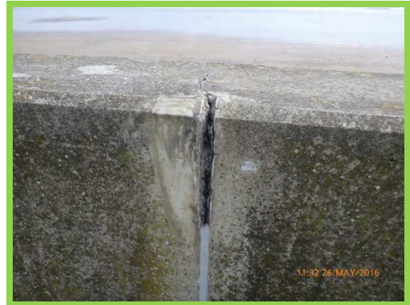
Loss of flexible joint sealant (/C0401C33)
