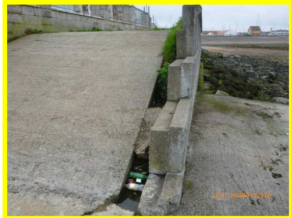
Void behind concrete wall units and beneath concrete ramp (/C0401C27)
