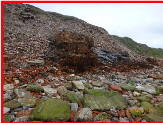
Potentially unstable remains of former gabion structure (/C0302C02)
