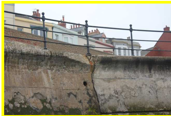
Damage to recurve concrete cope (/C0401C05)
