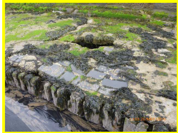
Void in apron of North Pier (/C0401C22)
