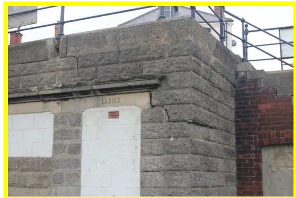
Cracking in former public convenience building (/C0401C05)
