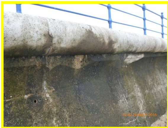
Local spalling of concrete (/C0501C05)
