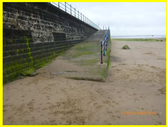
Foot of access ramp (Arabella Street) previously undercut (/C0303C01)
