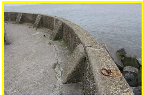
Cracking in concrete parapet wall and deck. Gaps between 'buttresses' and wall (/C0401C34)
