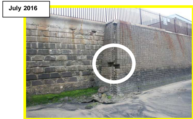
Missing blocks at interface between two walls. Local scour at toe (/C0401C19)
