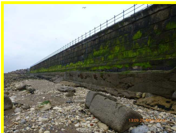
Damage to toe protection (/C0303C02)
