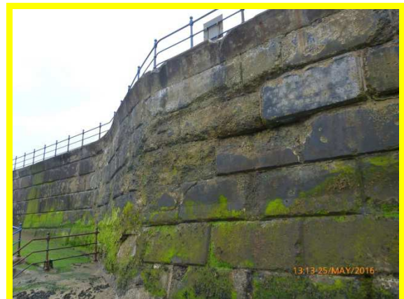
Spalling of concrete face (/C0303C02)
