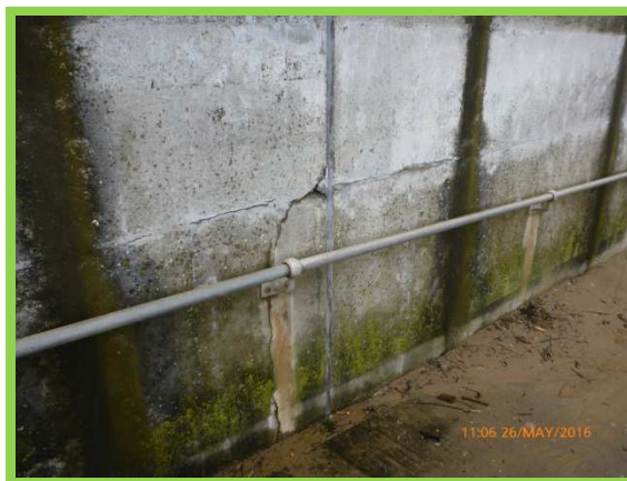
Cracks in concrete seawall at Little Scar access ramp (/C0401C33)
