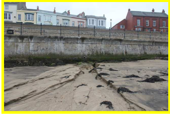
Local scour in front of outfall (/C0401C05)
