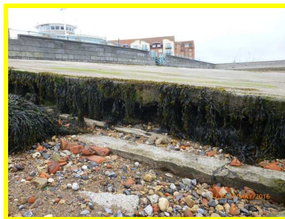
Undercutting of slipway (/C0401C27)
