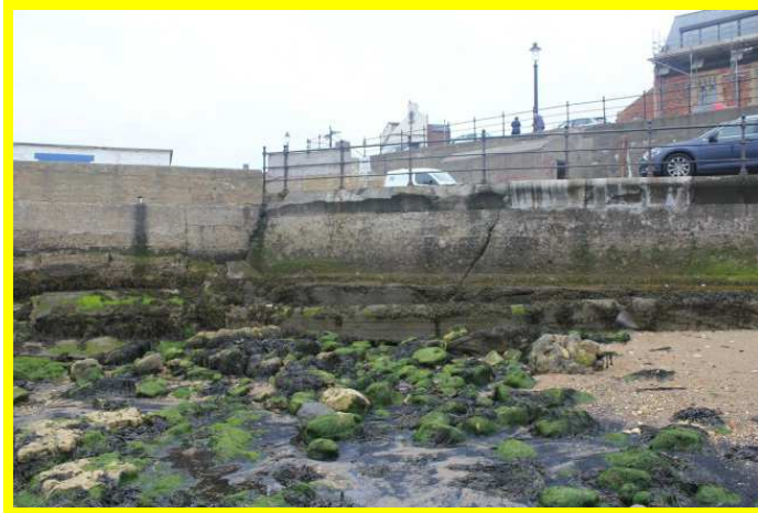
Undercutting and significant crack suggesting settlement. Old Pier to left of image (/C0401C05)
