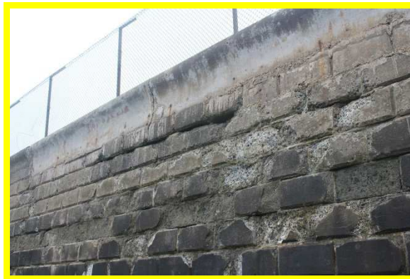
Spalling/abrasion of concrete blocks (/C0401C19)
