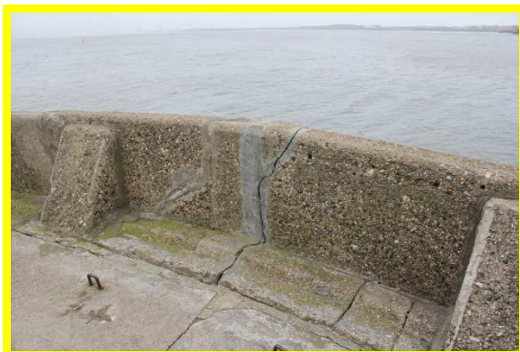
Cracking in concrete parapet wall and deck (/C0401C34)
