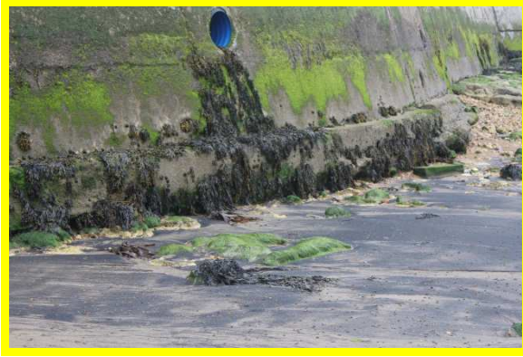
Undercutting – partially obscured by vegetation (/C0401C04)
