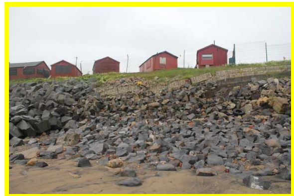
Settlement in stacked gabion wall (/C0401C17)
