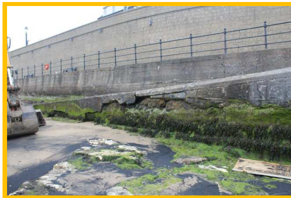
Voids beneath concrete deck of slipway (C0401C35)
