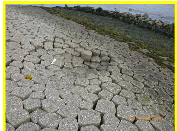
Local settlement of concrete blocks (/C0401C26)
