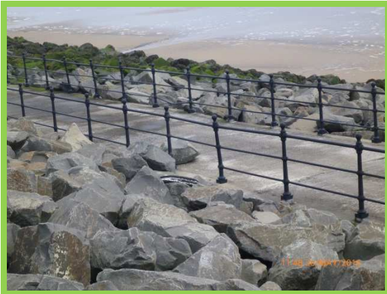
Displaced rock armour and damaged guardrail at northern access ramp (/C0401C33)
