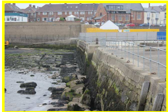
Inner face of North Pier – note potential settlement of masonry blocks (/C0401C06)
