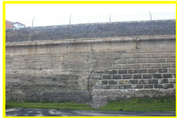
Vertical crack through parapet and seawall (/C0401C19)
